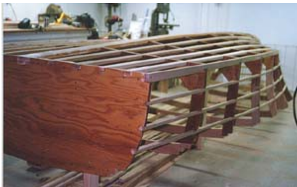
Fig. 3 - Stringers (longitudinals) are notched into frames and wrapped around the hull to support and stiffen the planking, and provide backing at planking joints.
