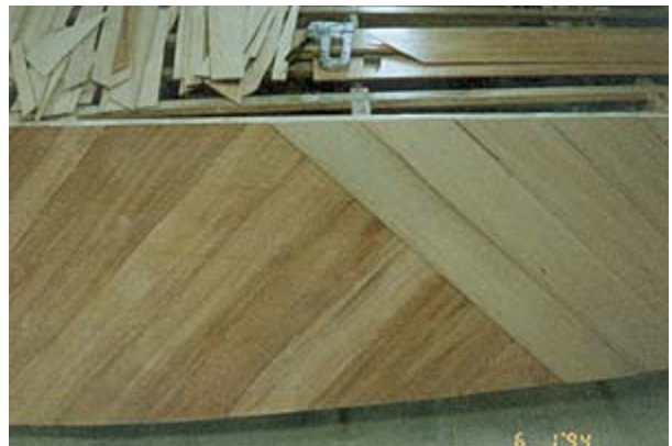
Fig. 4 - Planking from thin plywood or wood veneers is cut into strips narrow enough to comply to framework contours and applied in double-diagonal format to the prescribed thickness. Epoxy resin is used for bonding throughout. Fastenings can be temporary types at this stage.
