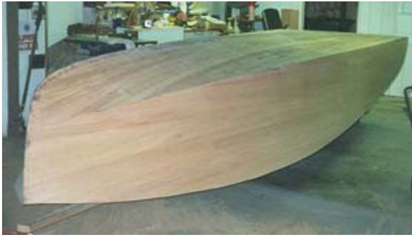
Fig. 5 - Final planking layer is applied lengthwise to emulate traditional planking of the past. John did the bottom this way also, but double diagonal format here is optional as well. Hull is now ready for fiberglass cloth & epoxy sheathing as provided in our FIBERGLASS COVERING KITS .
